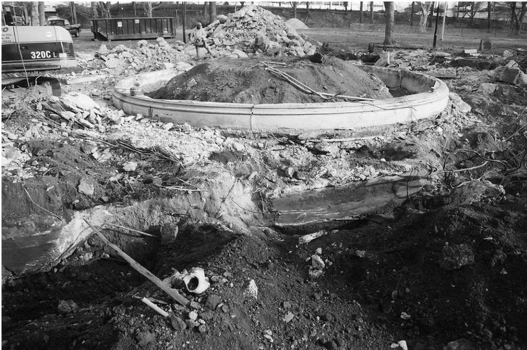
Plate 3. Demolition of fountain footers, view west-northwest. Note concrete footers with subsoil matrix, in foreground.
