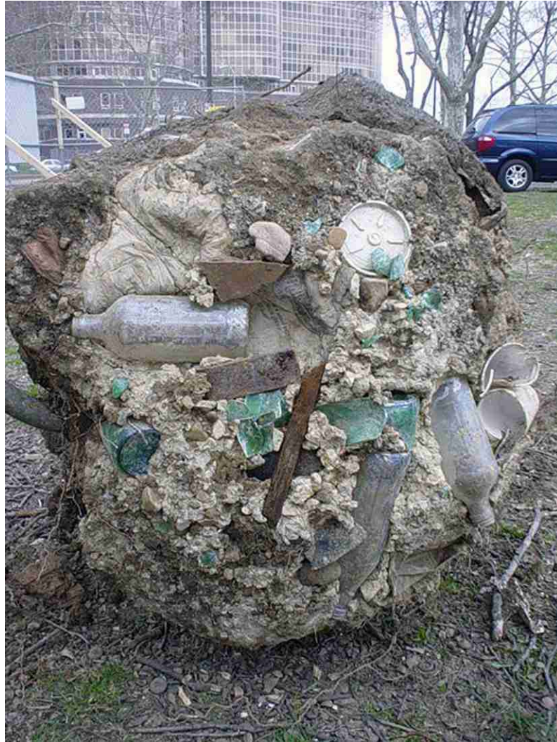
Plate 6. 1976 trash within concrete base of lighting standard in southwest corner of Franklin Square, view west.
